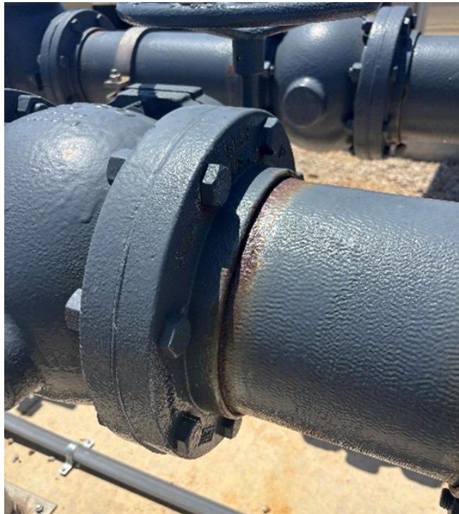
Figure 4-1: Visible Rusting of pipes
