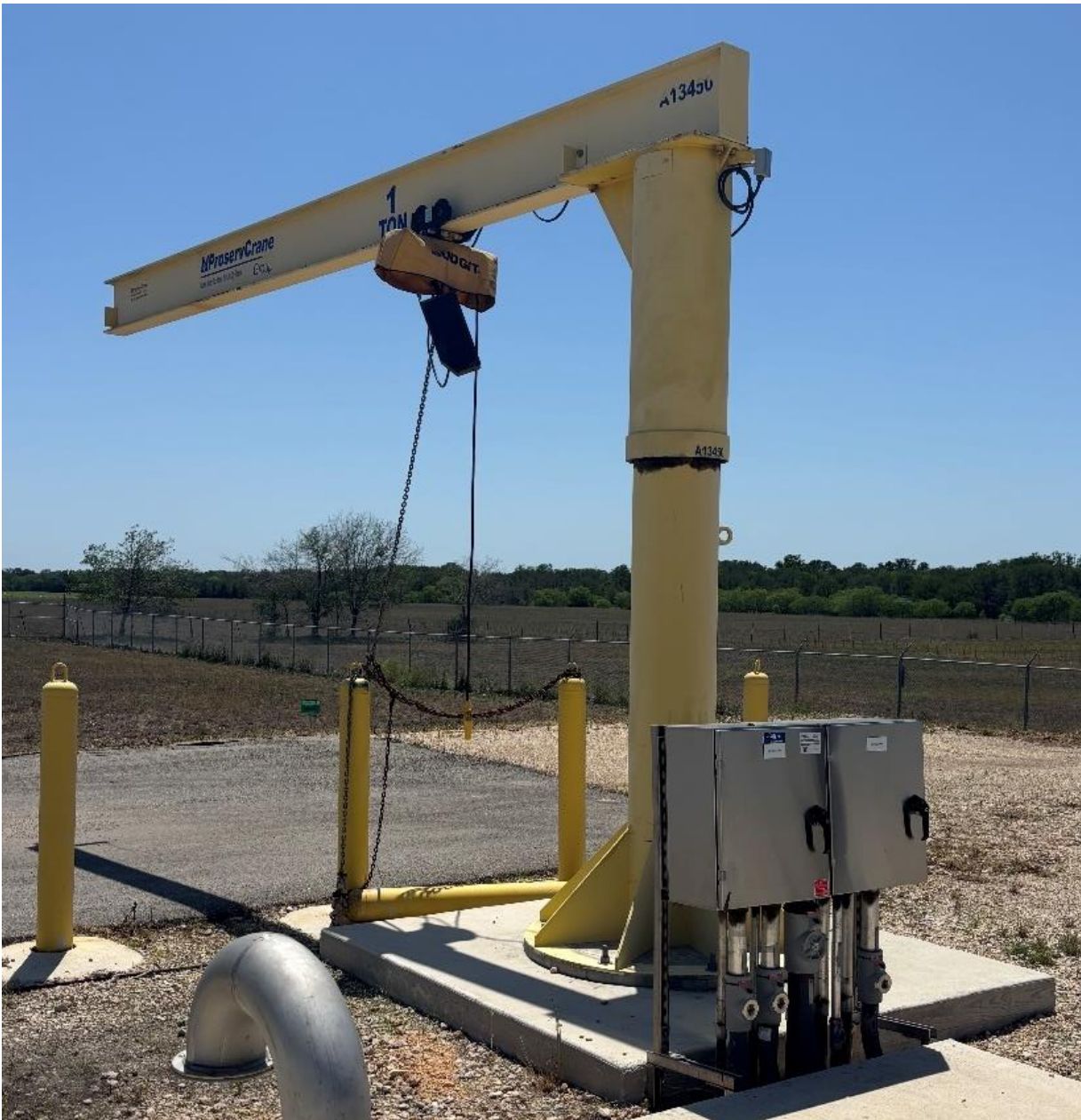
Figure 4-2: Jib Crane at Santa Clara WWTP
