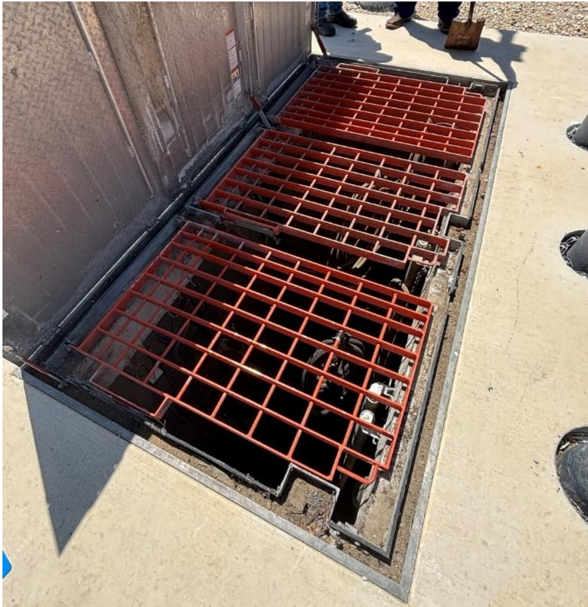
Figure 4-3: Santa Clara WWTP Influent Lift Station
